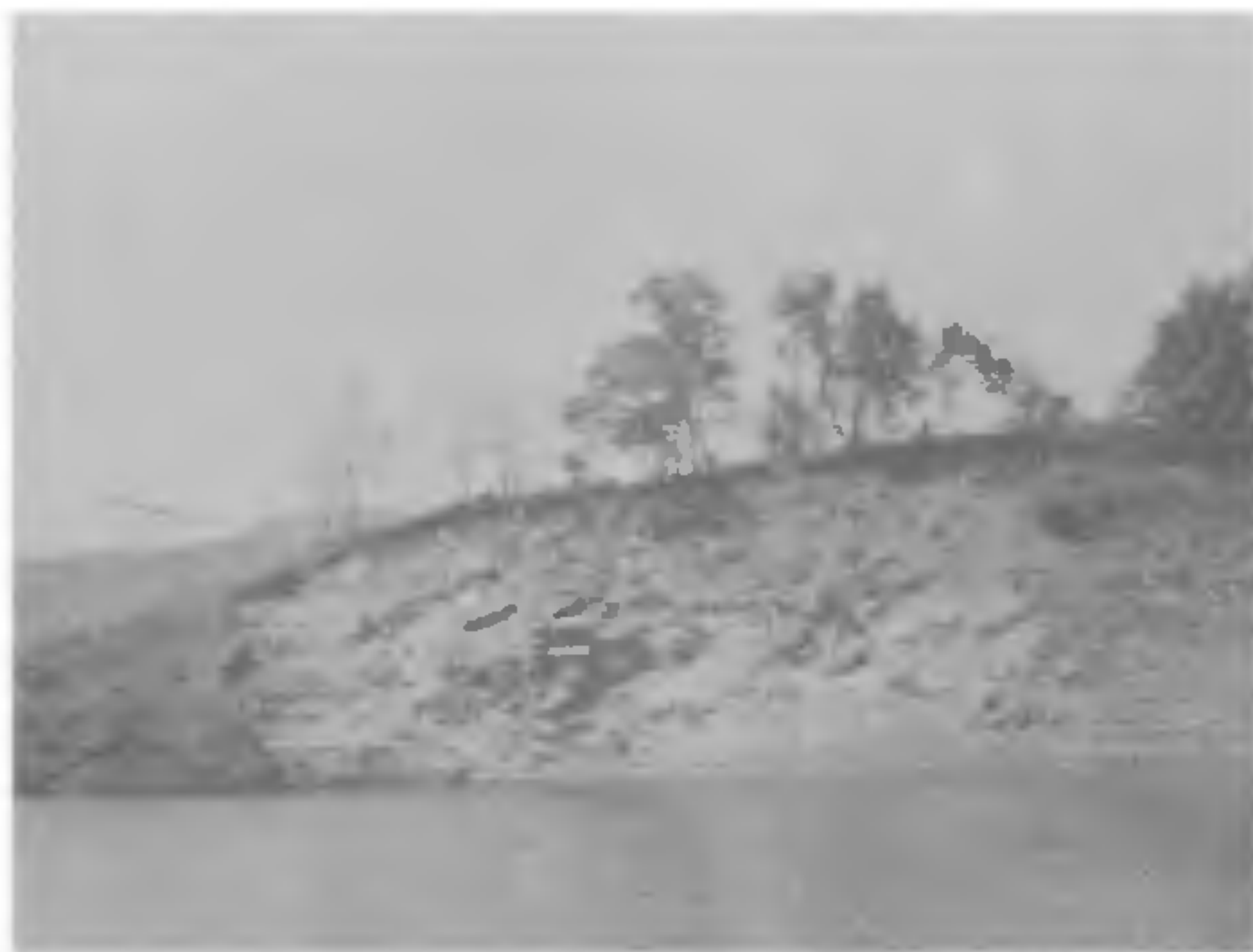
Figure 3. A major slumping in Periyar arm of the Idukki reservoir. The terracing on the slope is the result of beach action of reservoir water at different periods of lowering.
