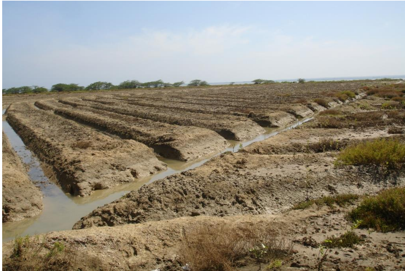
Figure 4. A typical canal system established in the degraded areas for regular flushing by tidal water
